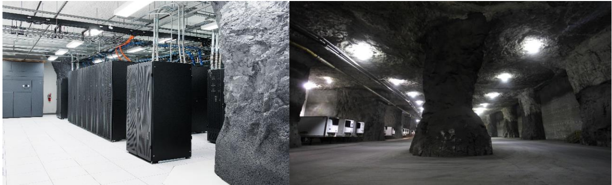
Fig. 16. Data processing center in the American Springfield, Missouri in an old underground limestone mine - DATA CENTER COMPANY EXPANDS UNDERGROUND IN MISSOURI [10]
