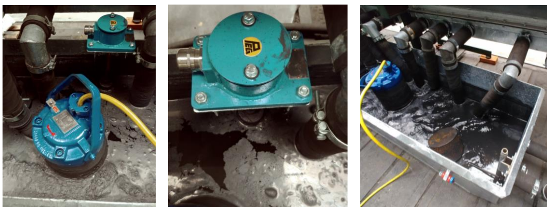
Fig. 8. The main components of the tank: water pump, water level sensor and float (tank condition after 30 min of operation)
