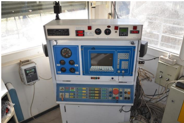
Fig. 11. The mixer controlling panel
