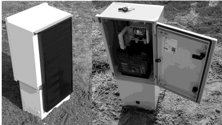
Fig. 2. Measuring station with photovoltaic power supply system used in the second series of tests
